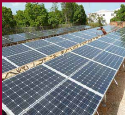
Solar installations at the Hughes Medical Centre: top - roof-mounted, bottom - ground mounted. Photo: ARIEP
